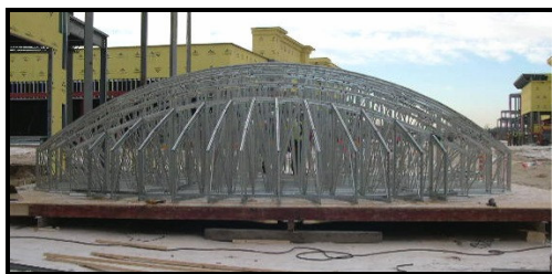
Picture of a circular roof assembled on a temporary platform prior to sheathing being applied.
