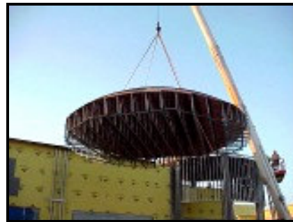
By locating the hoisting points for the crane, the contractor made one lift from the ground to the top plate.
