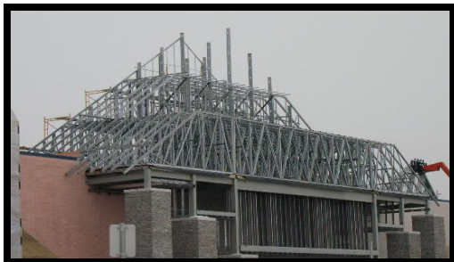
Exterior view of main entrance to Wal Mart with the "triple-decker" sections installed.
