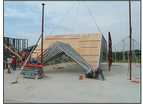
Truss assembly, with plywood sheathing applied and ready for lifting, weighed over 9,000 pounds.
