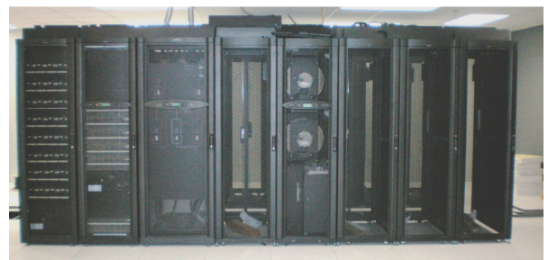
A row of server racks in the ITS data center
